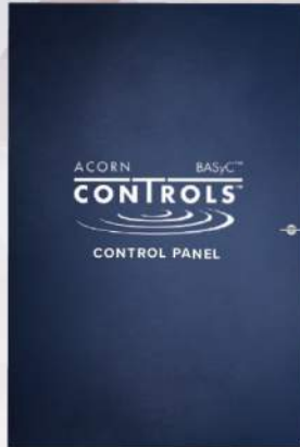
BASyC Control Panel
