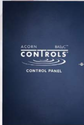
BASyC Control Panel
